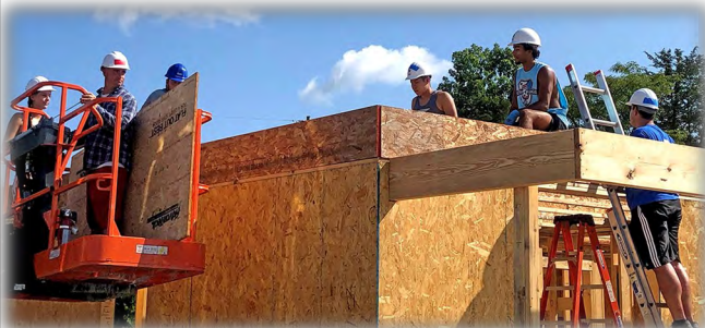
MTSU students in the Medical School Early Acceptance Program, or MSEAP, helped with a Habitat for Humanity build in Murfreesboro as part of their summer bridge week at MTSU. Nineteen students are in the program to help increase the number of primary care physicians serving medically underserved populations as well as alleviating health care disparities in rural Tennessee. (Submitted photo)
