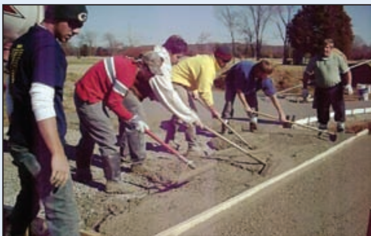
CLEARING A PATH —Concrete industry management students work to level concrete poured for a golf-cart path at Champions Run. Making the effort are, from left, Ben Kurdy, Sean Freeman, Seth Williams, Jackson Ballman, Will Flanigan and Ed Kowalski.
