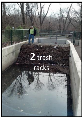
Trash rack in the Murfree Springs Wetlands
